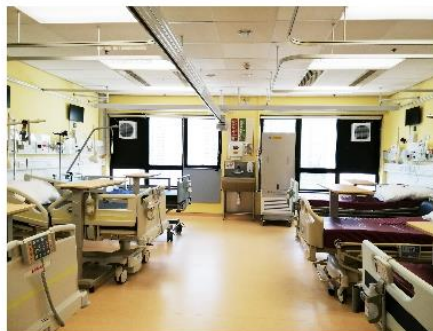
Two additional exhaust fans are installed for every 6-bed cubicle of each ward
