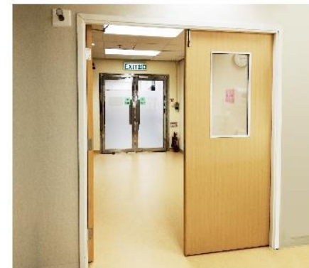
Additional door installed at the entrance of ward creates a buffer zone which helps stabilise the negative pressure inside the ward
